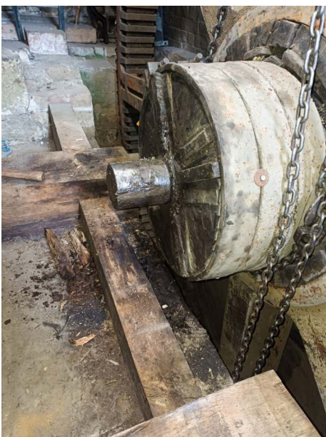
Plenty of clearance with broken beam removed
