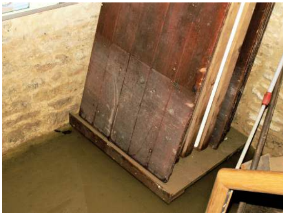
Tide mark on the stored tables in the waterwheel room
