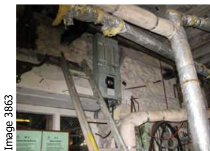
Board B - 3 phase distribution
