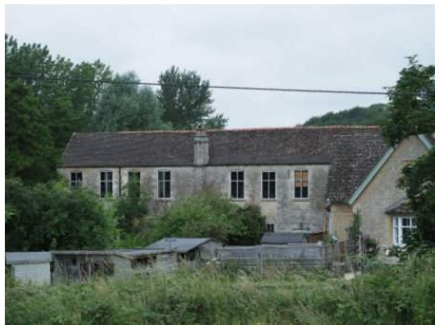
Field view of Mill showing tile coverage and absence of old slates on left hand face. All windows are new.
