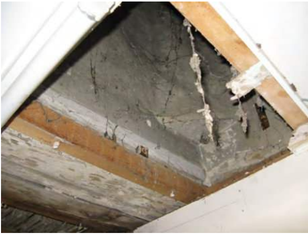
View into bell tower through hatch with left hand ceiling plaster awaiting replacement
