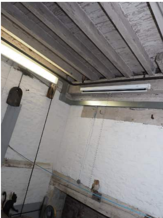
Pull down projector screen opposite Cornish Boiler
