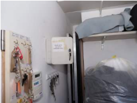
Key press mounted in bell turret store room
