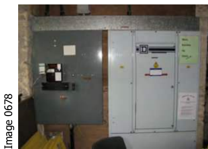
Board A - incoming 3 phase
