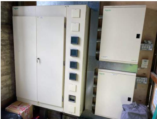
Main Mill distribution centre in Footmans' Bathroom on Second Floor
