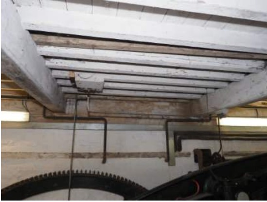
Electrical trunking (galvanised) run at ceiling level
