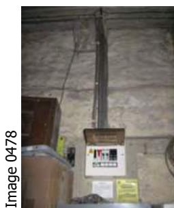
Board D - Mill ring main + lighting mcbs
