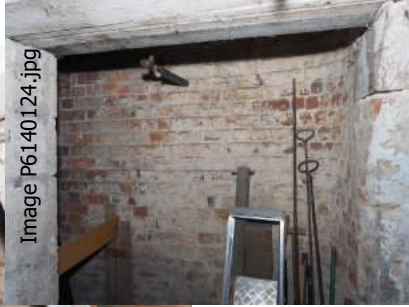
View into passage from front of Cornish boiler
