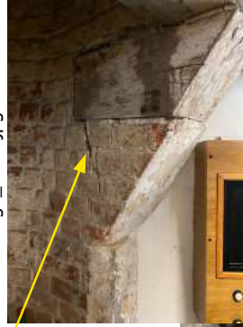
Crack in brickwork supporting beam
