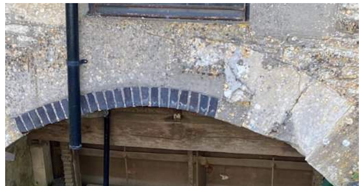
Headrace arch - slight indication of masonry crack being monitored
