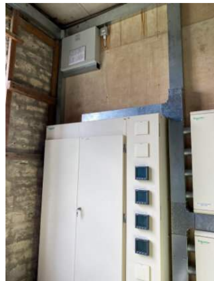
Control box upper left - intruder alarm (not used)
