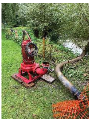
Our main river water pump failed and is away being repaired
