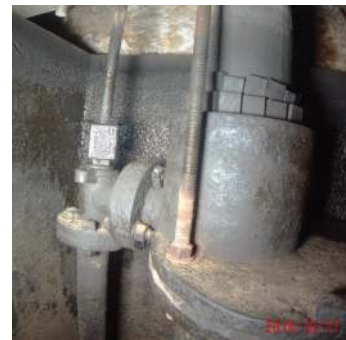
View of spray valve in the cold well
