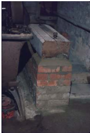
Plinth of outrigger pulley bearing
