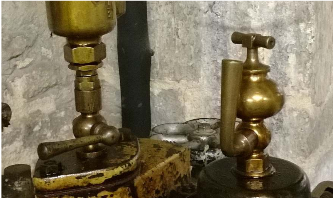
Figure 6 Reader Engine: Lubrication Valves Shown in their CLOSED Positions
