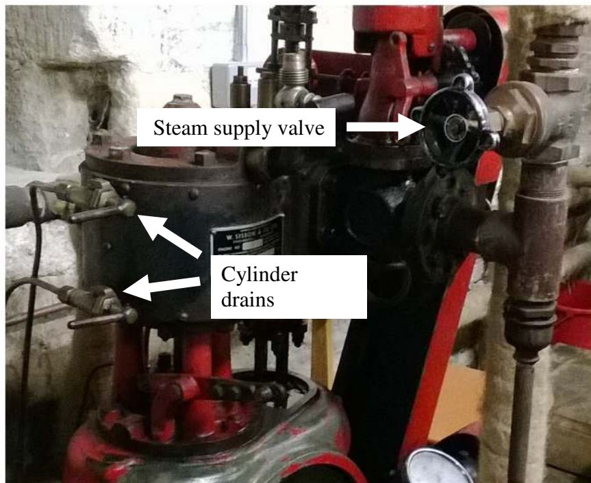
Figure 4 Sisson's Engine: Steam Supply Valve and Cylinder Drains
